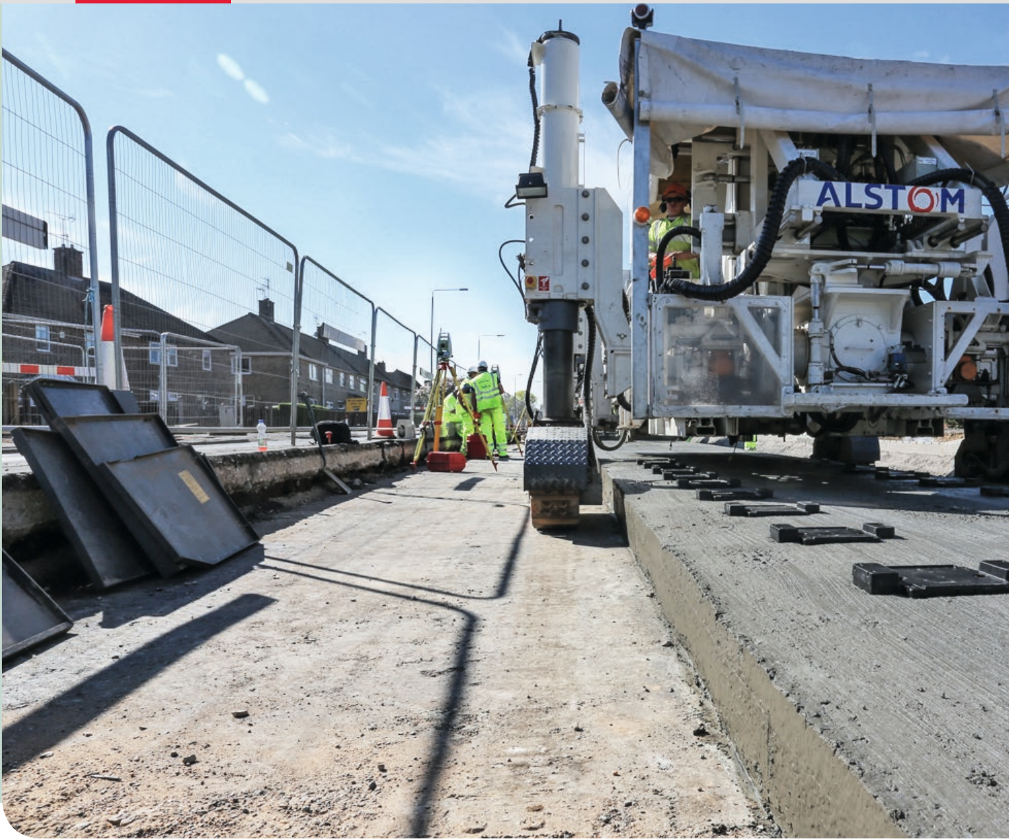
■ Guided by Leica Viva TS15 total stations and PaveSmart 3D, Alstom's Appitrack™ ensures a smooth tram platform.
