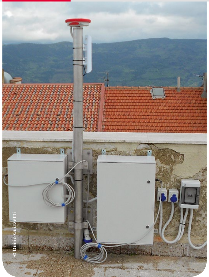
■ GPS Monitoring Station
