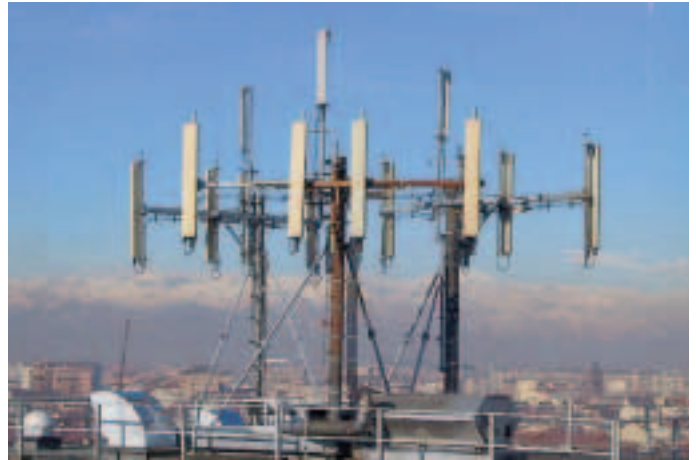
TIM Antenna site
