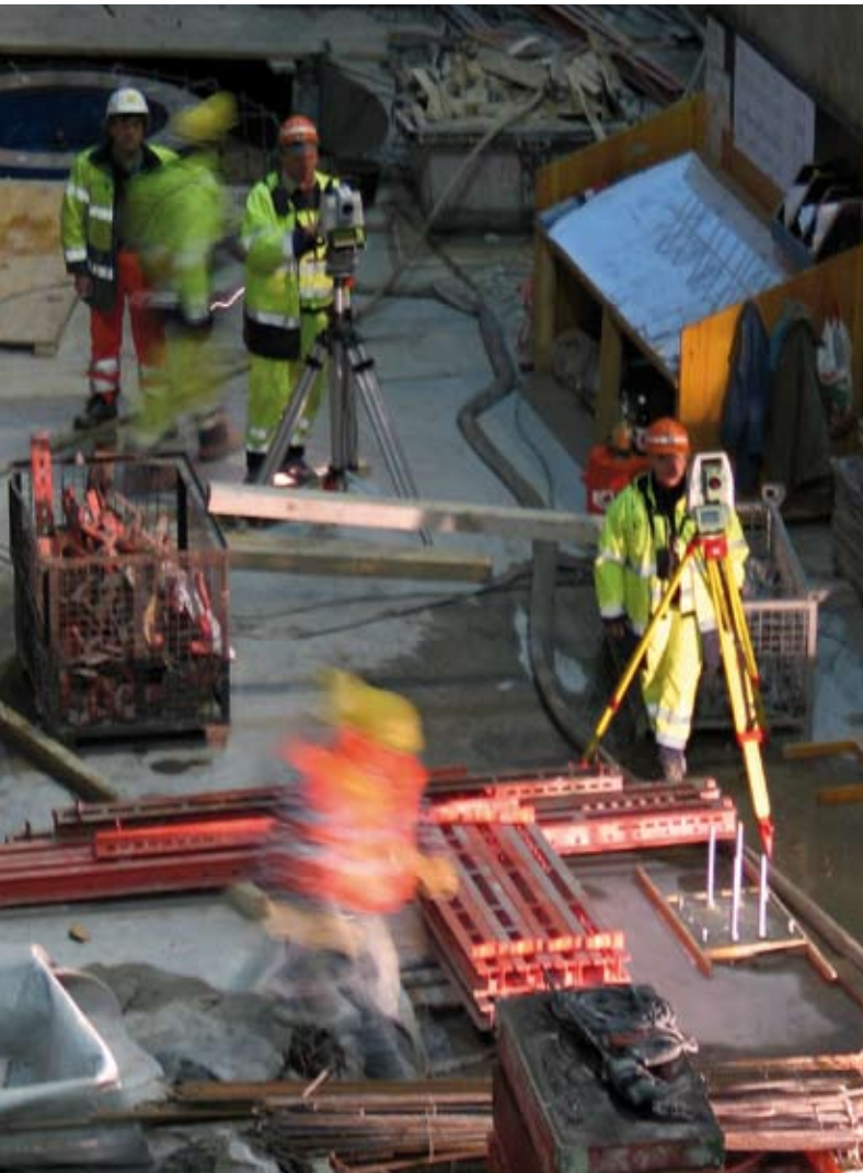
■ The cavern with its three machine towers will form the heart of the power station.
